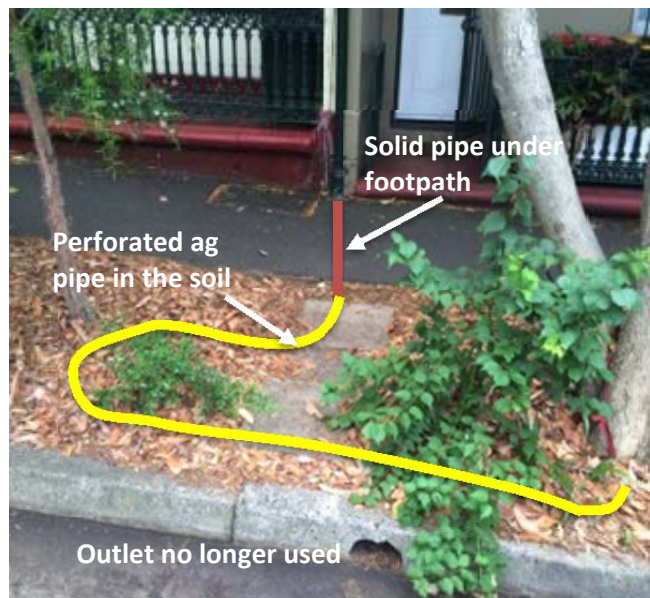
Figure 1: Photo showing approximate location of leaky drain in Myrtle St Chippendale
