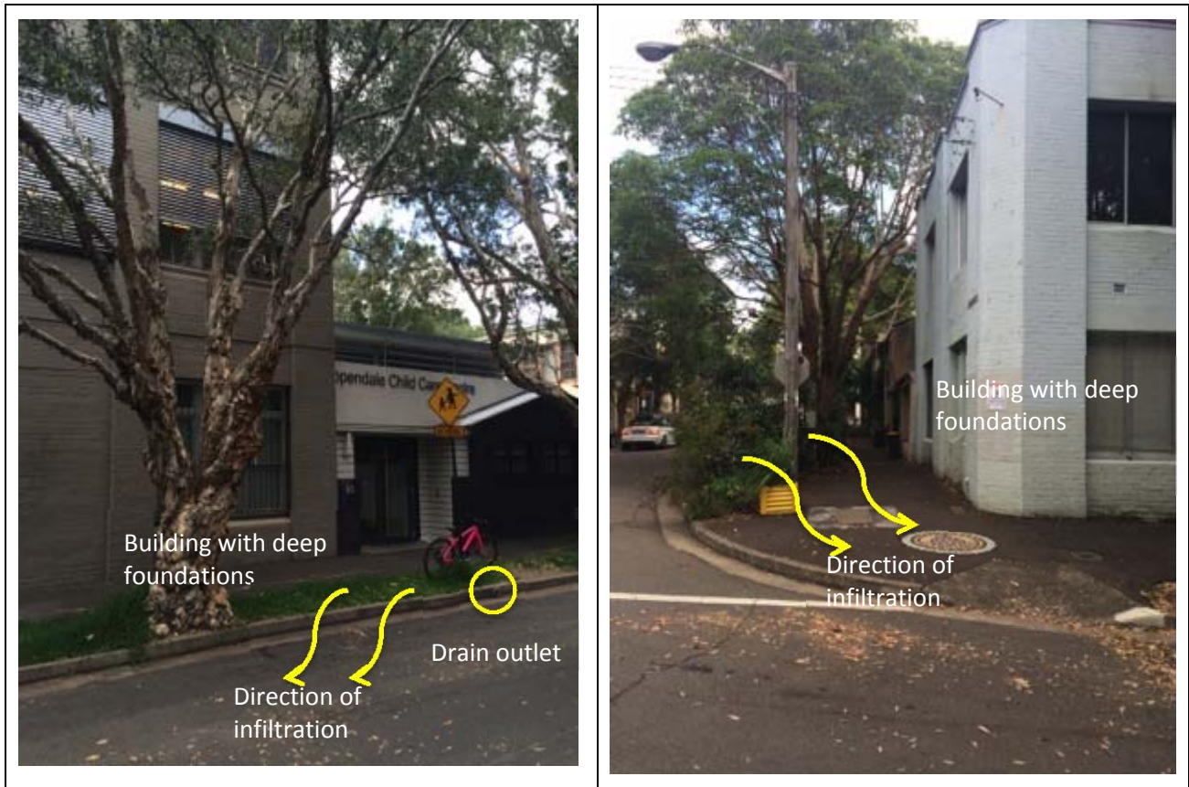
Figure 6: Showing two locations where infiltration may impact on the foundations of existing buildings.
