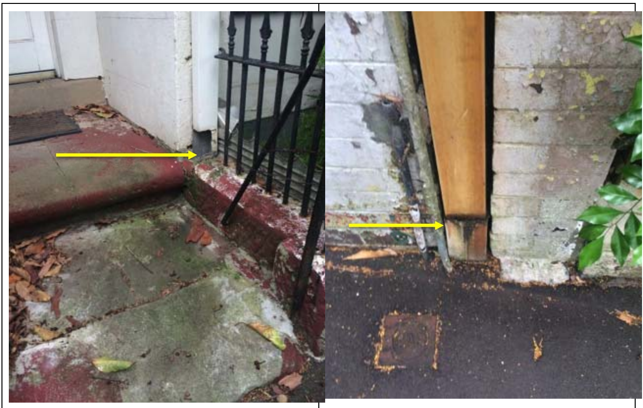
Figure 7: Downpipes in Myrtle St showing signs of neglect
